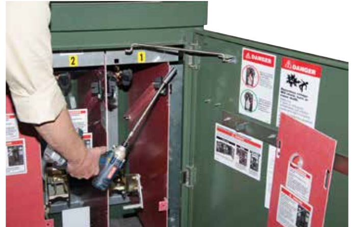
Figure 2. Preparing to remove roof retaining hardware. Note 9/16" socket on extension bar with wobble attachment and power driver. (Live-front design shown for illustration purposes only.)
