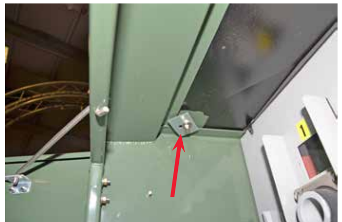
Figure 3. PSE clamping bracket in corner of termination compartment.
