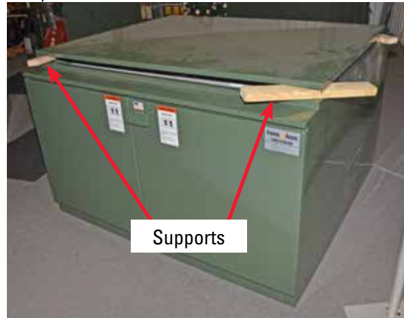
Figure 6a. The roof is supported on all four corners by blocks.
