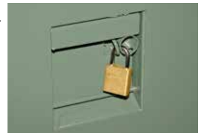
Figure 14. Always close, latch and padlock the enclosure door before leaving the unit or when working on the opposite side.
