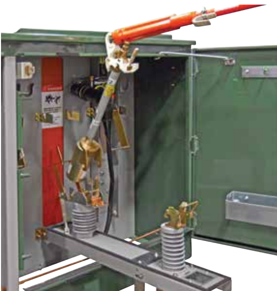
Figure 31. Shotgun clamp stick secured to fuse pull ring and fuse assembly being lifted from the latched position and being removed from fuse hinge.
