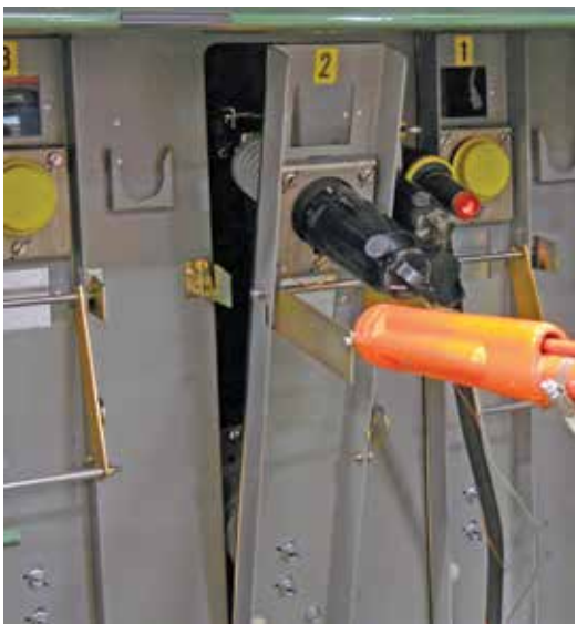
Figure 27. Fuse mounting being lowered to access fuse (or raised to reinstall fuse).
