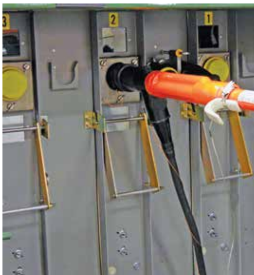
Figure 22. Shotgun clamp stick secured to elbow with elbow in process of being removed/connected to bushing insert.
