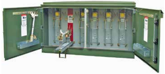
Figure 19. Fuse compartments with doors secured open.
