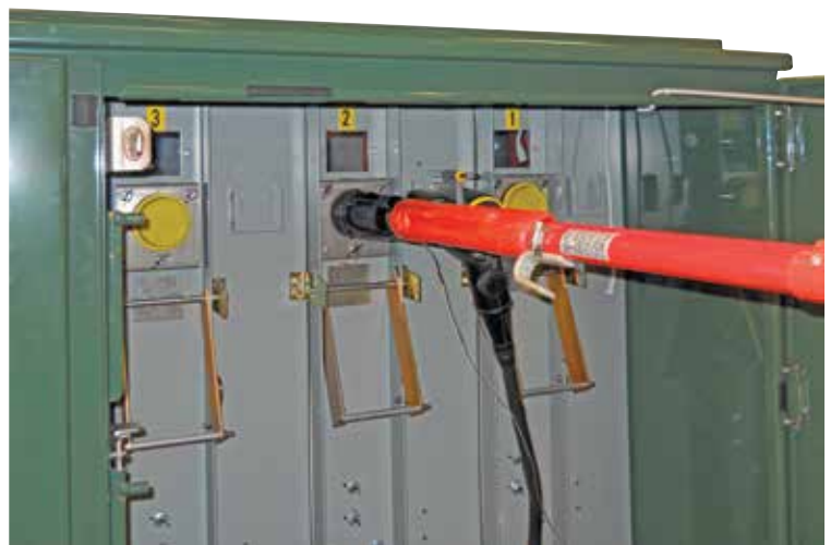
Figure 24. Insulating protective cover installed on bushing-well insert.
