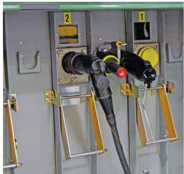
Figure 20. Feed through standoff bushing installed on parking stand.
