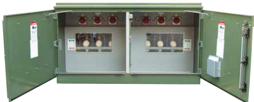
Figure 15. Visually verify switch position through switch viewing window. Viewing window orientation and position will vary depending on the specific unit design. Viewing window in termination compartment above is typical.
