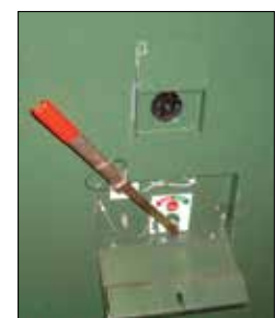
Figure 13. Alternate switch-viewing port and operating handle extended.
