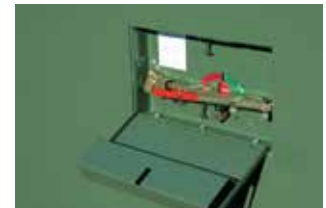
Figure 8. Open switch lockbox access cover. Handle is connected to enclosure by a cable.
