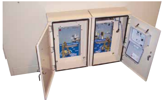
Figure 17.c. The Self-Powered Overcurrent Relay is in a weather-resistant enclosure and is mounted on the inside of the low-voltage compartment door that also includes the manual handles for operating the vacuum fault interrupter and the visible disconnect.
