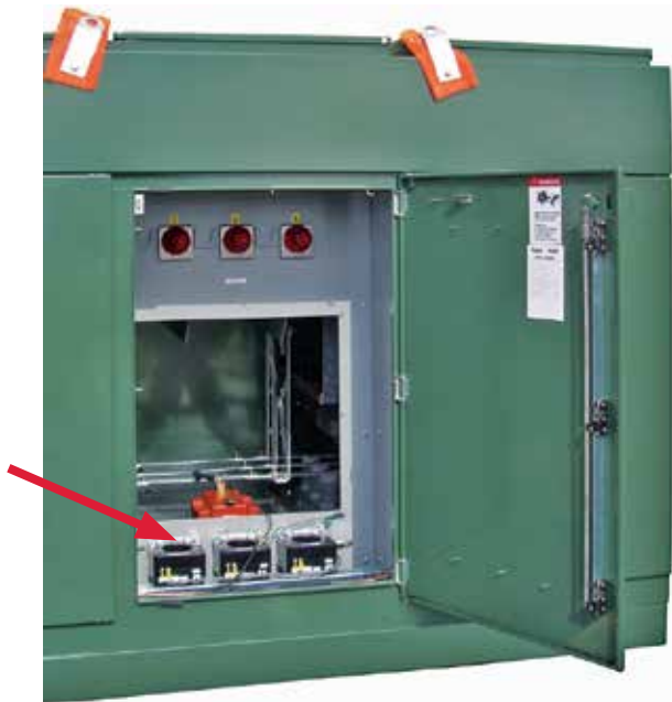
Figure 18c. This view shows an alternate location for a fused-voltage transformer (at arrow). In this installation the VT opening will be covered by a bolted steel panel that includes lifting handles. View also shows "bracket-supported" window-type CTs.
