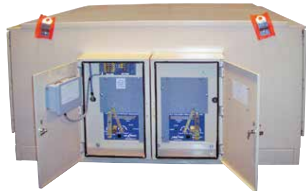
Figure 17.b. The Self-Powered Overcurrent Relay is pictured above installed in combination with Vacuum Fault Interrupter (at left) to provide overcurrent protection for a load feeder circuit. Vacuum Interrupter at right is manually operated and provides switching for the main-primary feeder circuit.
