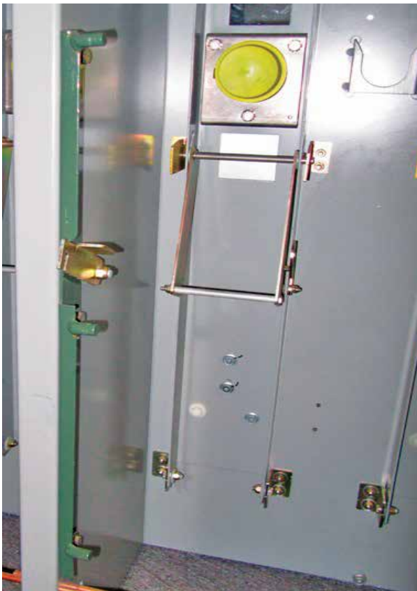
Figure 1 – The front of striker rail is mounted flush with the edge of center divider wall.
