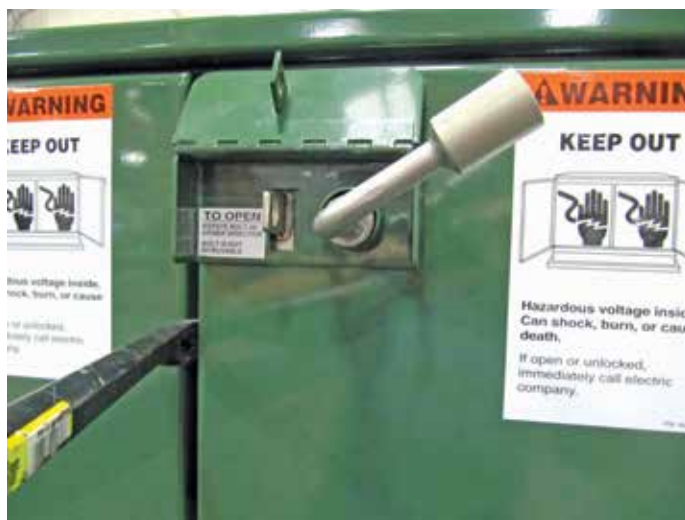
Figure 6. Prying the edge of the active door while applying tension on the latches.
