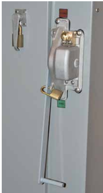
Figure 18. Key interlocks on manual switch-operating handle to guard against possible undesirable paralleling and to prevent opening the door unless downstream switches are open.
