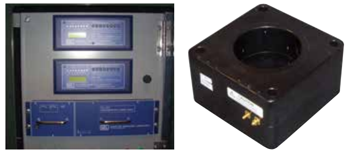
Figure 11. Overcurrent Protection is provided using The SEL-501 Dual Universal OCR (see above left). Each OCR relay control can handle two vacuum fault interrupters. A UPS (at bottom in above left photo) is included to make certain control power is always available for operation of the relay to trip the vacuum fault interrupter in response to a fault a UPS is included. A current transformer (see above right) is used to sense the overcurrent condition and provide that input to the SEL-501 relay.
