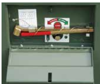
Switch-Operating Handle Storage
