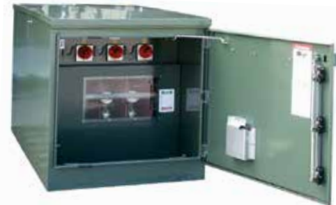
Switch-termination compartment of a dead-front SCADA Controlled unit is pictured above.
