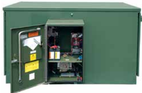
Motor operator on SCADA Controlled unit of pad-mounted switchgear.
