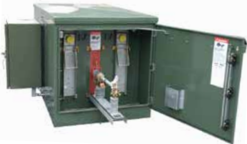
Fuse compartment of dead-front SCADA Controlled unit is pictured above.
