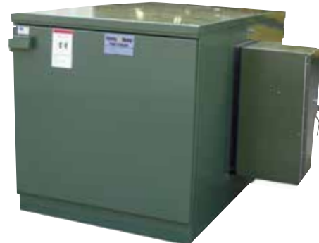
Motor operator allows remote operation of switch.
