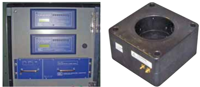
Figure 11. Overcurrent Protection is provided using The SEL-501 Dual Universal OCR (see above left). Each OCR relay control can handle two vacuum fault interrupters. A UPS (at bottom in above left photo) is included to make certain control power is always available for operation of the relay to trip the vacuum fault interrupter in response to a fault a UPS is included. A current transformer (see above right) is used to sense the overcurrent condition and provide that input to the SEL-501 relay.
