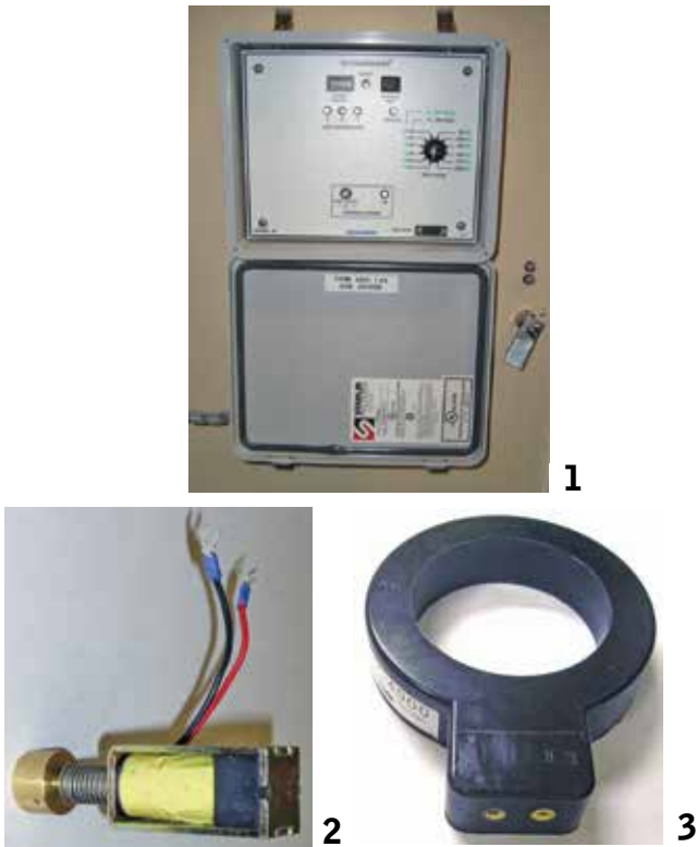
Figure 10. The self-powered relay components include (1) the relay that provides all the settings and controls necessary to initiate vacuum circuit-breaker operations based on the programmed parameters, (2) the magnetic actuator pictured that provides mechanical trip-actuation of the vacuum circuit-breaker mechanism and (3) the current-sensing transformer that provides sensing and power input to the relay and trip circuit.
