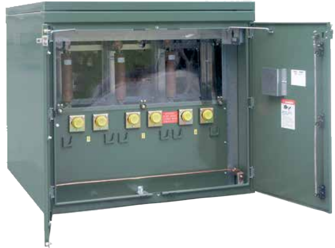
Figure 8. In this dead-front capacitor bank, the current-limiting fuses are visible through the optional clear polycarbonate barrier (suffix-B6).
