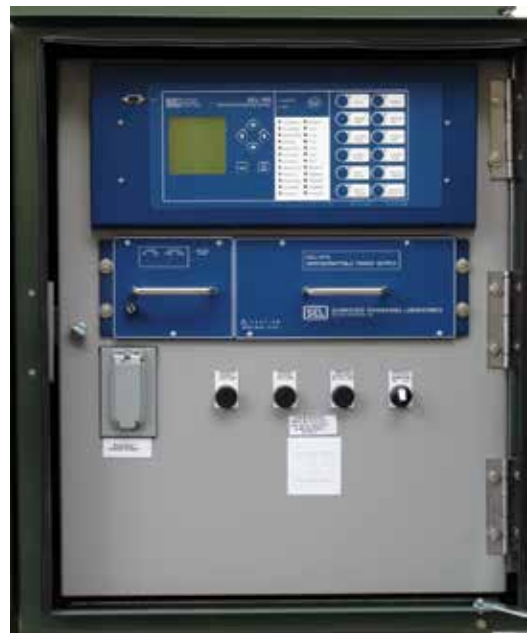
Figure 6. Controls for MAVRiC® units equipped for automatic source transfer utilize the SEL-451 preprogrammed with Federal Pacific software developed to provide all the functionality, including field programmable timer settings, and voltage and current level pick up and dropout settings. MAVRiC® utilizes magnetically actuated vacuum interrupters so that motor operators are not required for automatic transfer operations to be performed. In addition to the capability to operate both MAVRiC® units even when one power source is lost, the control package for automatic source transfer includes a UPS to insure that control functionality is maintained even when both sources are lost.
