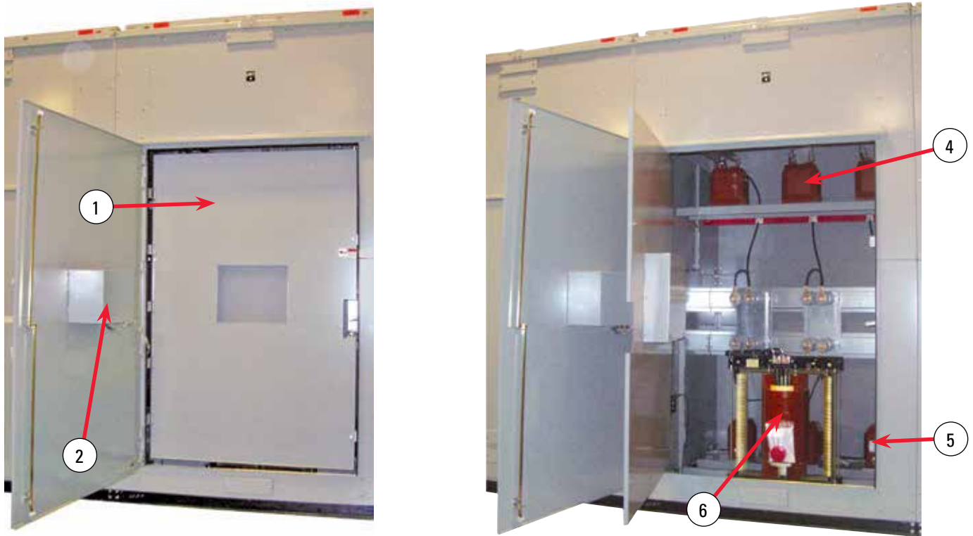
Figure 7. Bay 4 — The Customer Metering Bay with an Advanced Metering Relay is pictured above and in inset below.
