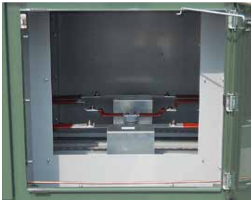
Figure 7. This is a close-up view of the interior of Compartment 5 through the panel opening. The steel support plates visible in the bus at the bottom of the switchgear metering unit are temporary bus supports which will be removed and replaced by the bar-type CTs, to be installed by the customer.
