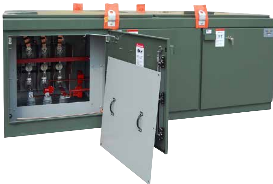
Figure 5. The access panel of Compartment 6 is shown removed, providing views of, and access to, the internal bus and the incoming 600-ampere loadbreak switch in the medium voltage compartment.
