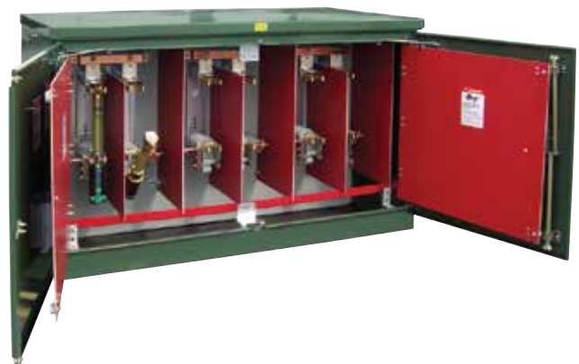
Figure 4. The FUSE compartment is pictured with the barriers secured open and showing one set of two fuses on the left phase – one fuse is latched closed and one fuse is shown in the disconnect position. The fuse mountings are non-loadbreak so the elbow has to be used to break the load current, de-energizing the circuit, before disconnecting the fuse.
