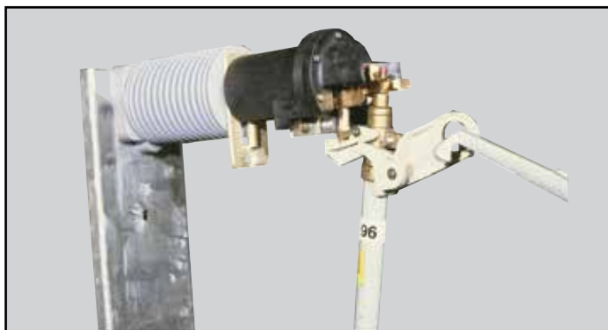
Figure 2. Main Contacts Have Parted, Puffer Spring Charged, and Interrupter Parted.
