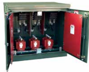
Metering Transformer Compartment With Barriers Secured Open
