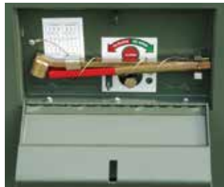
Switch-Operating Handle Storage
